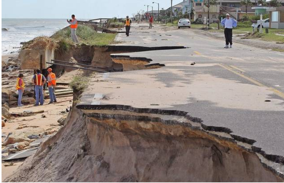
Figure 4: Damage to the AIA in Flagler Beach from beach erosion caused by storm surge and high waves. Courtesy: Miami Herald.
